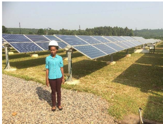
Figure 5. Kalangala Renewables' solar PV array. Photo by Energy 4 Impact.
