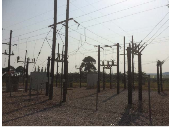
Figure 4. Kalangala Renewables' substation. Photo by Energy 4 Impact.
